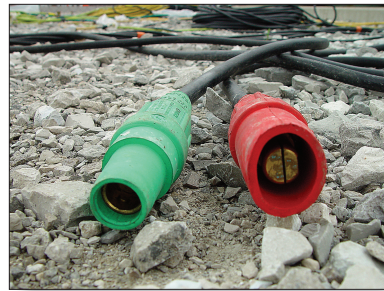
Figure 2.23 Cam-lock connectors. Thick cables (often one or two aught thick) are used to supply the needed power. Often a single truck can draw more than 100kW. These cables can have more than 100A flowing through them. Users twist the cam-lock connector to lock or unlock it, which creates a slight scraping action that cleans the mated surfaces with each use. Very little dirt, read resistance, is required to cause heat buildup and arcing when so much current is flowing. Heat buildup and arcing causes carbon buildup, which creates more resistance and ultimately the cycle leads to failure, or at least unreliability in the connector. One more thing, never pull one of these cables apart while the truck is under load. Besides the fact that the truck's EIC and other people using the truck will not like you, the arc caused by high current as the connector is pulled apart could destroy the connector. You might not like the result of that destruction either.
