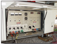
Figure 2.22 Power bay with three-phase 208V power with no grounding
