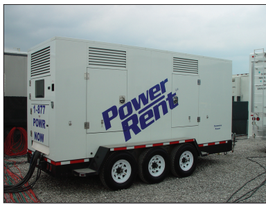
Figure 2.24 Often backup power generators are rented.
